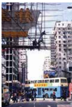
Fig 4: This bamboo structure needs the wall and not the other way around. (Photo supplied by Serge Gracovetsky private correspondence)
